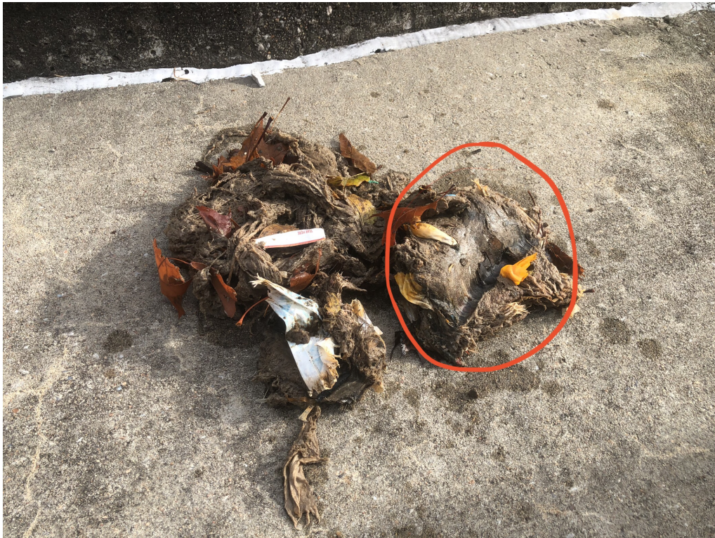
Clog from RAS Pump
